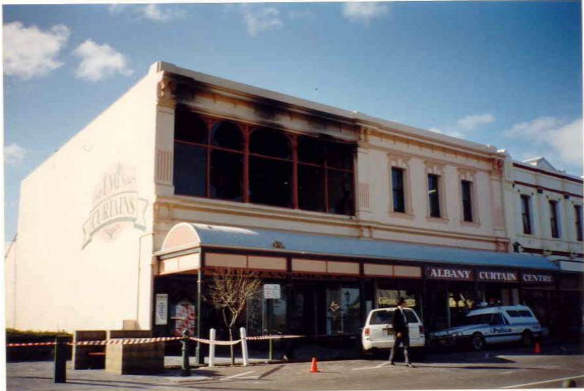
Fire damage to upper storey 1999.
