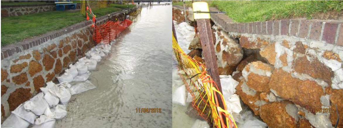
Figure A1-7 Photographs from April 2012 showing damage to the original 'brick wall' seawall at Oyster Harbour Beach (Source: URS, 2012).
