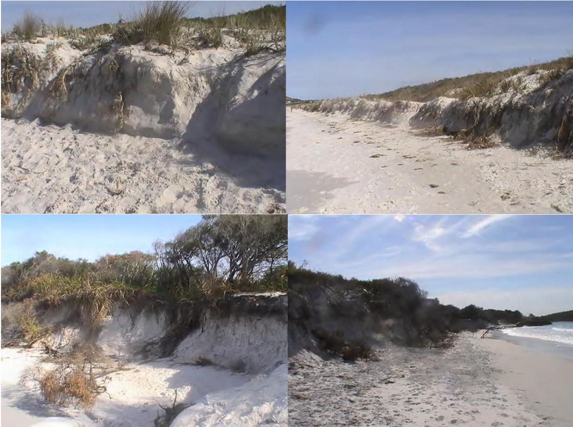
Figure A1-5 Photographs from 2012 showing the smaller erosion scarp (source: URS, 2012)
