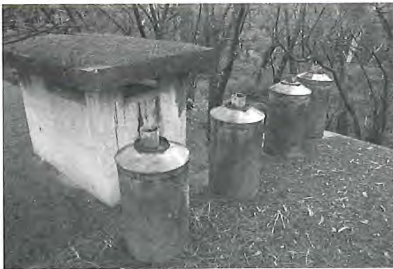
Engine Exhausts [City of Albany, 2010]
